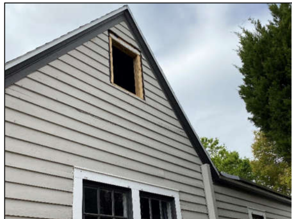
Figure 4: Missing unit on February 21, 2020.
